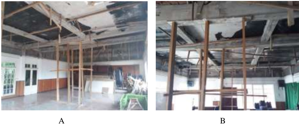
Figure 4. Structural reliability condition A and B. Damage is in the beam components located in the hotel conference room (deflection and cracking).
