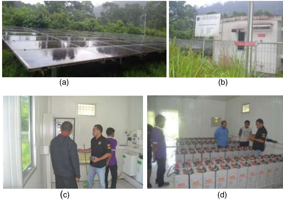
Figure 6. Solar power system of Alue Keujrun village (a) solar cell after cleaning, (b) power house, (c) panel control inspection (d) battery bank inspection
