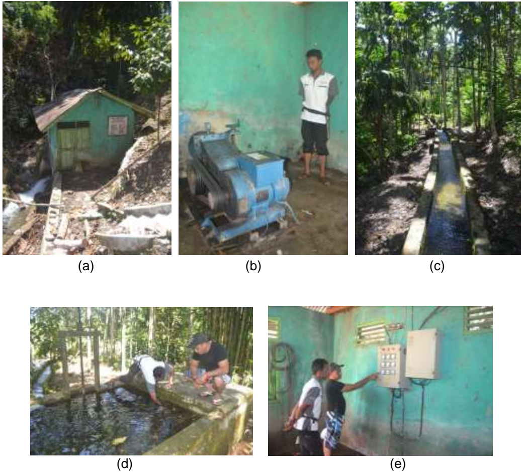
Figure 7. Hydro power system of Alue Keujrun village (a) power house, (b) power generator, (c) panstock, (d) forebay cleaning, (e) control panel and dump load
